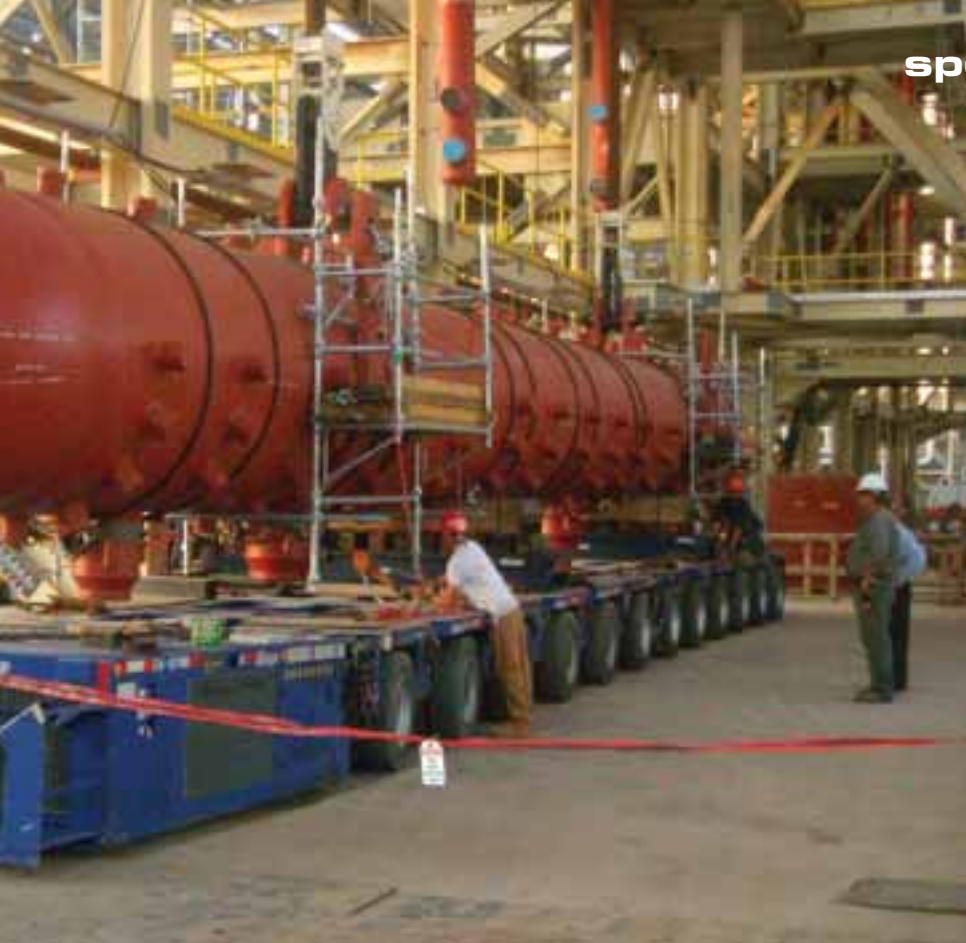
The scope of Bigge's work at the plant involved lifting boiler components, including steam drums and boiler modules. Bigge first set the two 190-ton steam drums using a pair of strand jacks mounted on top of the boiler steelwork to lift the drums 165 feet to their final elevation
