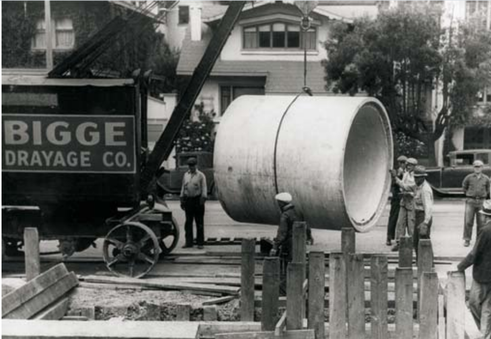
The first crane built by Bigge was used to lay the main water and sewer pipelines in the City of Oakland during the 1930s.
