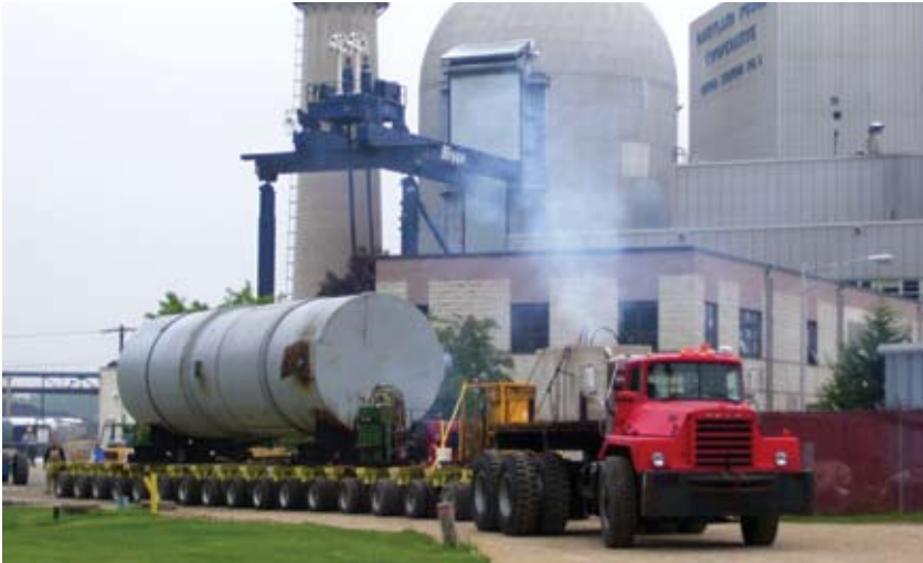
Engineered, managed and executed through-the-hatch removal, lift and transport of a reactor vessel (RV) from containment.
