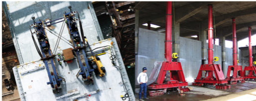
Above left: Strand-jacks were used to lift linkspan deck sections on San Francisco's new Bay Bridge across Oakland Bay. Bigge proposes the same system for removing falsework.
