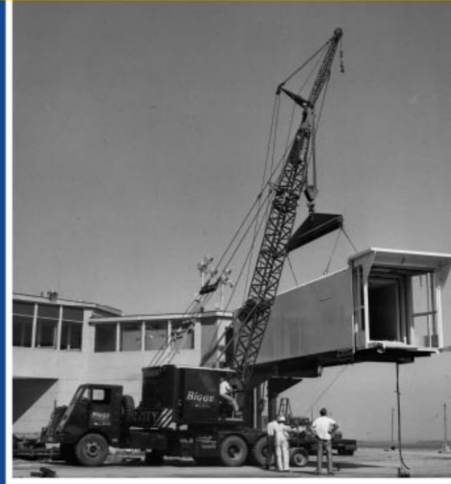
S.F. International Airport Hauling and erecting jetways for Pacific Iron & Steel Corp.
