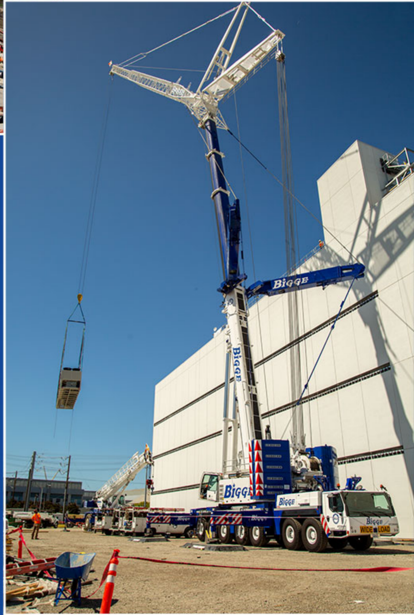
Data Center Cooling Units Santa Clara, CA
