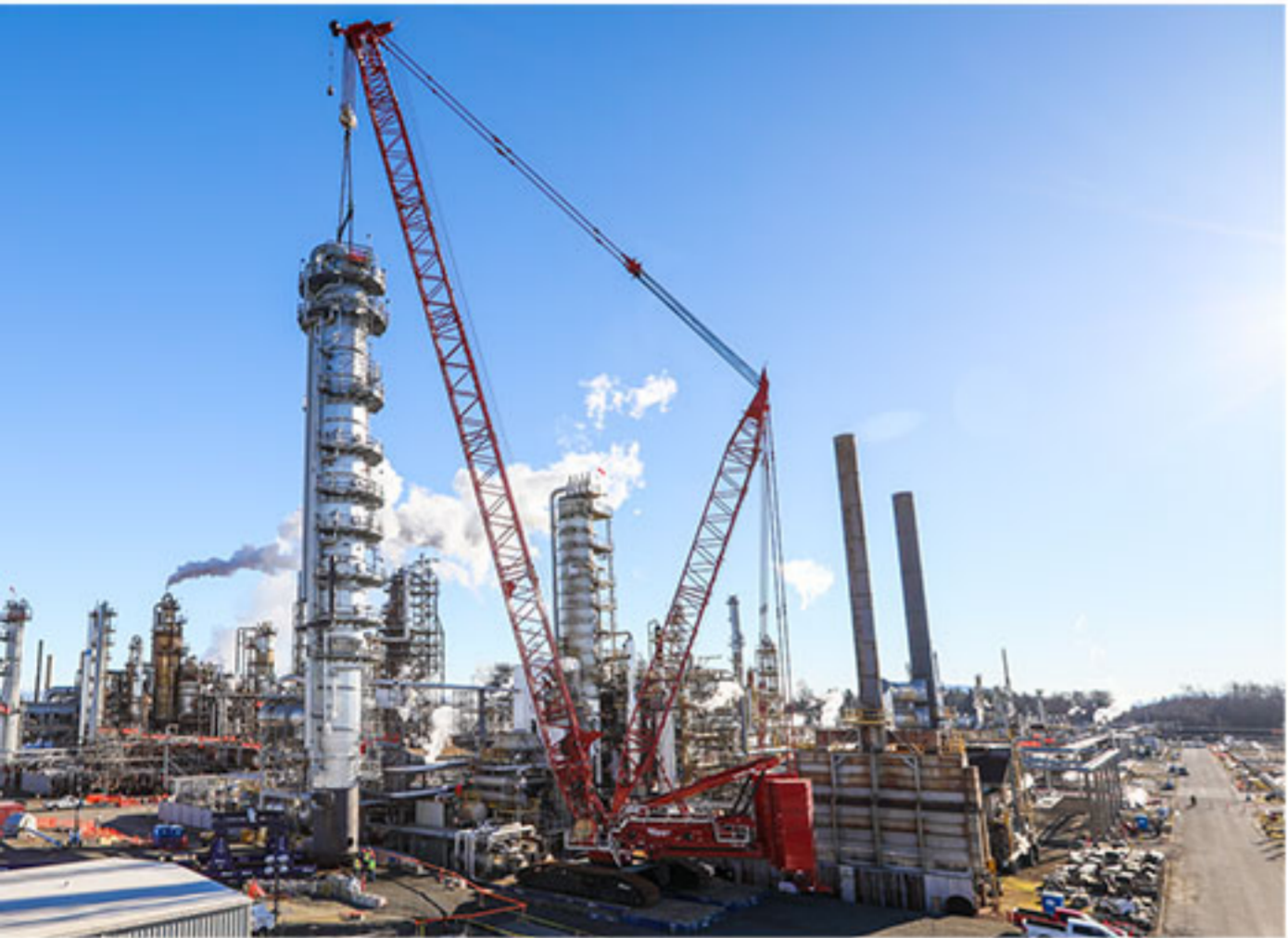
Refinery Vessel Washington
